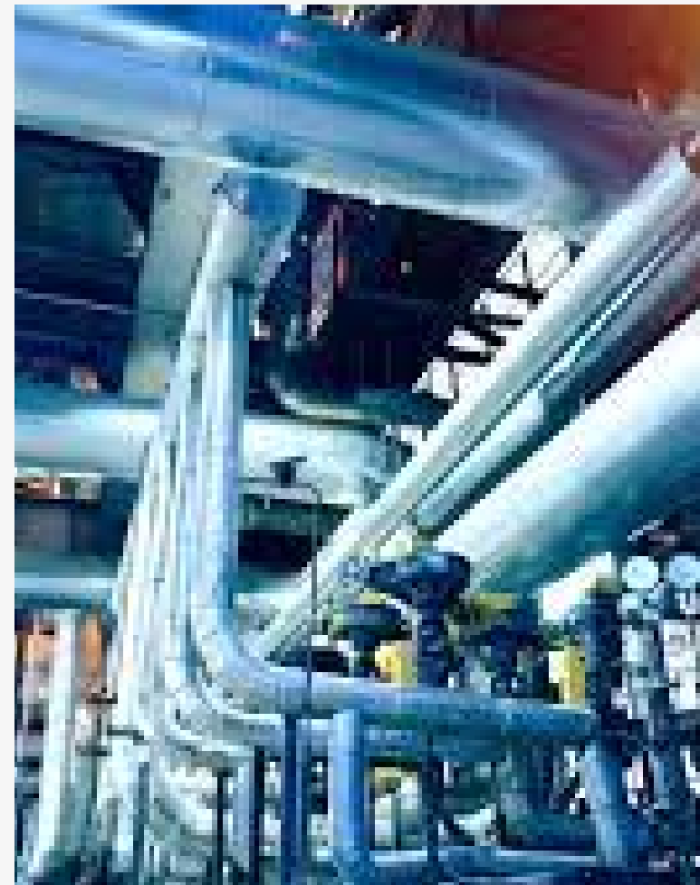
CONTROLS AND AUTOMATION SYSTEMS
